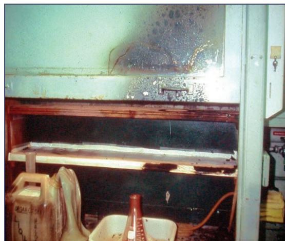
Figure 5. Aftermath of a hood fire.
